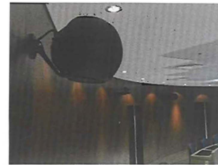
EV Evid 4.2 wall-mounted speaker in the auditorium
